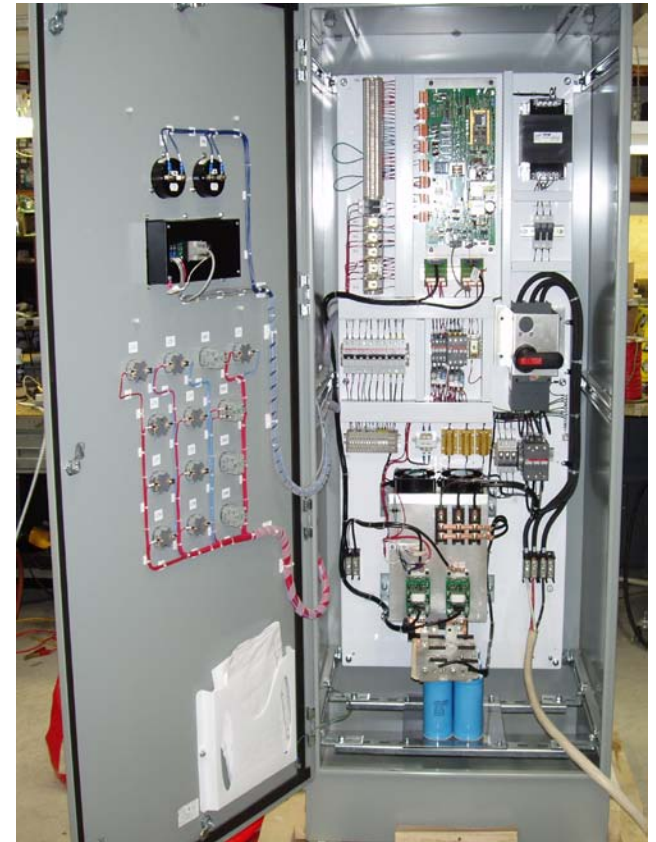
Mid Frequency 400Hz Power Supply Control Cabinet
