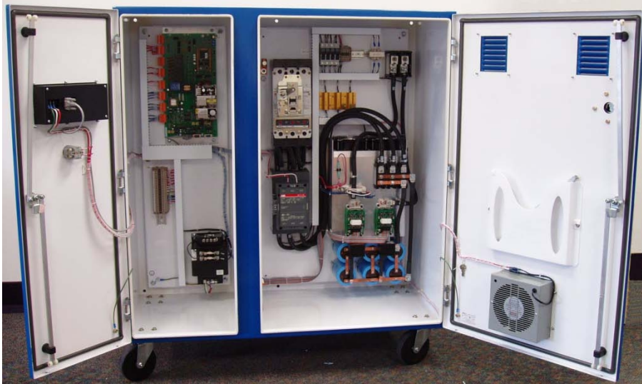
Mid Frequency 400 Hz Power Supply Control Cabinet
